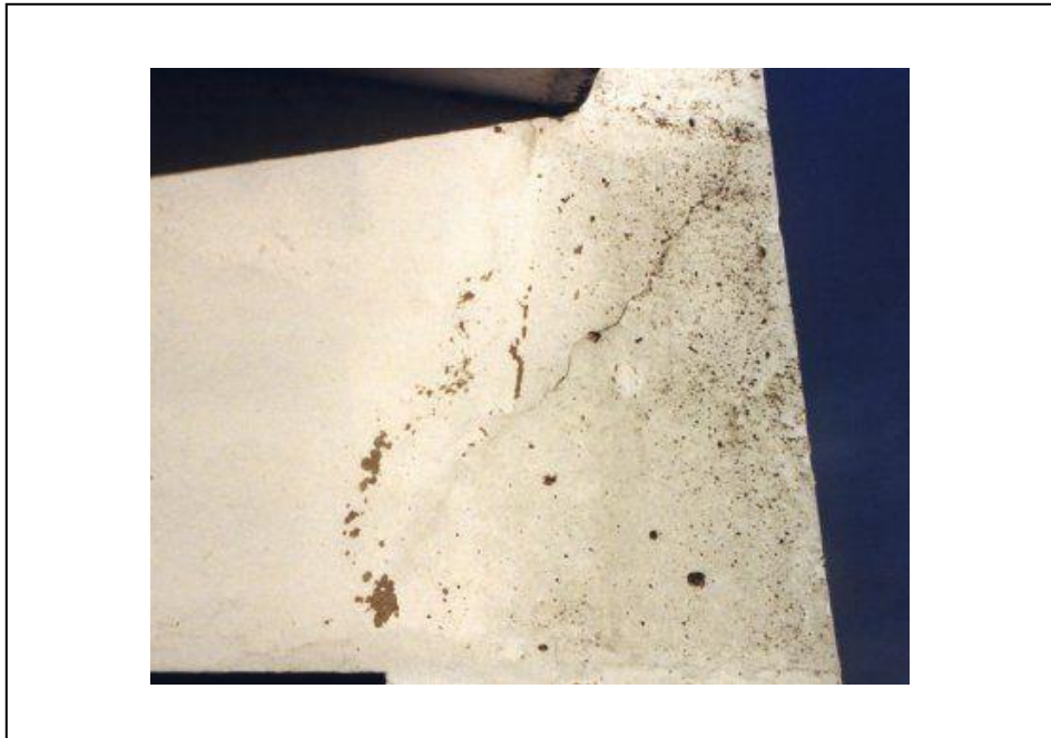
Figure 3(a) Cracking within an external beam-column joint - photograph
